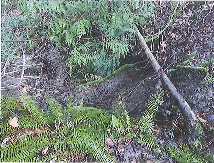
Photo 11. View north over the upper end of head cut below Wetland I (5/4/22).
